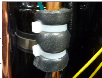
Figure 6: Thermistor attached to the refrigerant line.
